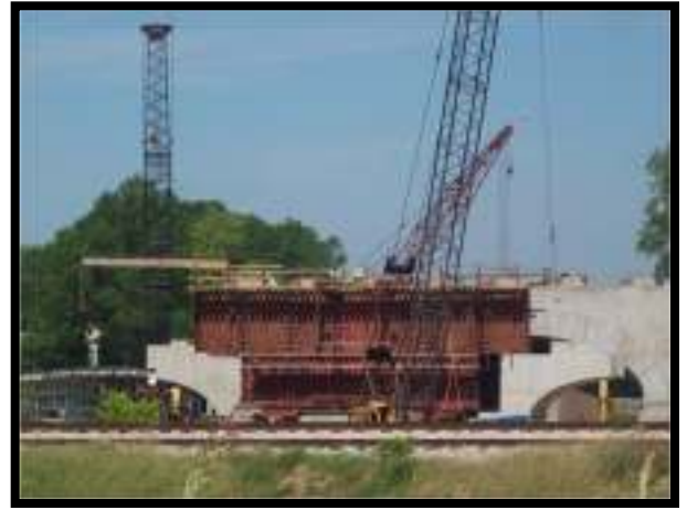
Shown is one of the support structures for the new elevated highway under construction in Madison.
